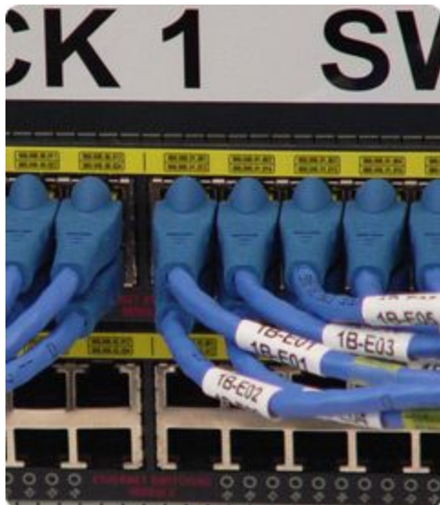
Labeled ethernet cables
